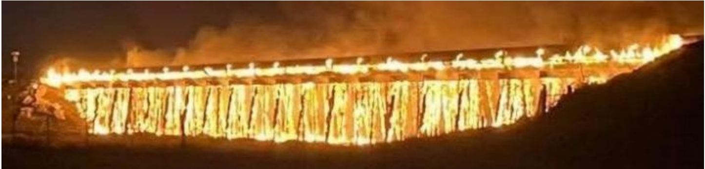
A still from a video showing the BNSF trestle outside of Canyon, TX ablaze. (Photo by Amarillo Fire Dept.)
